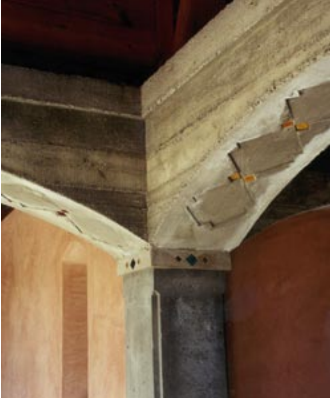
▲ Cast-in-place concrete column and arch with lacquered copper inserts give authenticity and rustic elegance to the interior.
